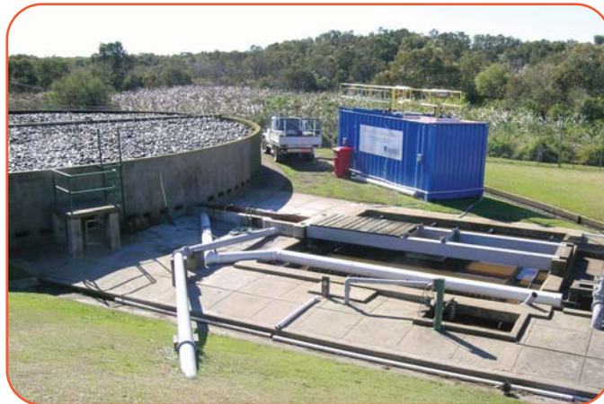
Fig 3. ViroSewage™ Technology containerised mixing and dosing plant alongside trickling filter.
