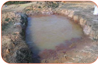
Water contained in the pit shown above was also treated using ViroFlow™ Technology
