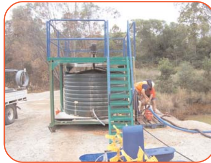
Photo showing Acid B Extra™ reagent mixing and dosing plant and aerators in the foreground.
