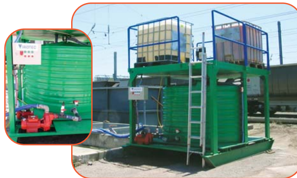
The ViroFlow™ Technology plant which treats waste water with ElectroBind™ reagent.
