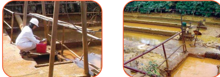
Figure 4 & 5. These concrete channels were the input to the lime treatment plant in Baia Mare. Two mega litres of AMD water was transferred from this plant to a containment dam that was used to test the Acid B Extra™ reagent.
