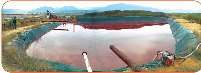
Figure 6. This pond was constructed to conduct the Acid B Extra™ reagent AMD treatments in Baia Mare. The pond was lined with geosynthetic liners and contained 2 ML of water.
