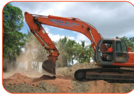
Mixing ViroBind™ reagent with contaminated soil at the Ross River site using an excavator.
