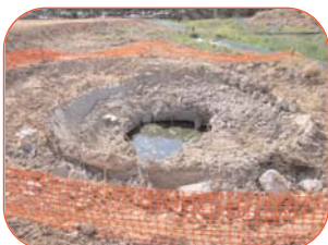
Underground sludge tank
