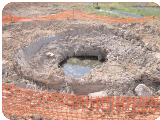
Figure 1 - The underground sludge tank at the CMC site
