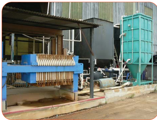
Figure 1: View of installed water treatment system
