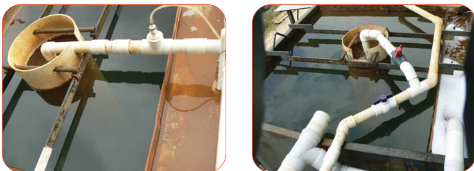
Figure 2: Clarifier tanks (right and left)
