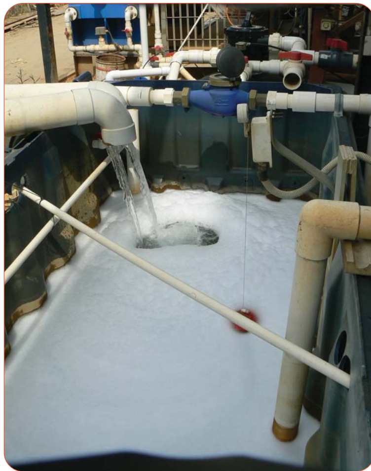
Figure 4: Treated water discharge
