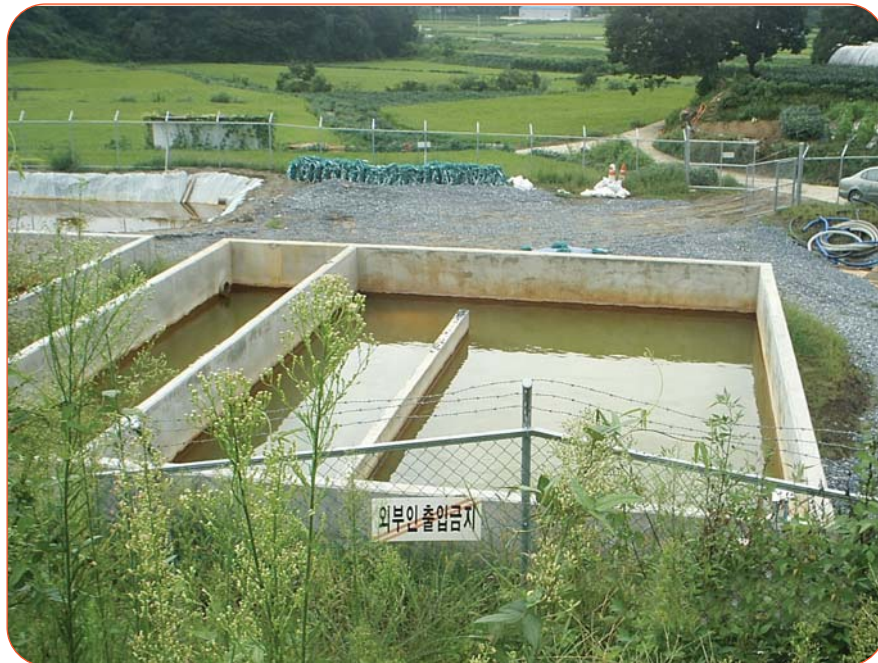
Figure 6: The ViroMine™ Technology filter system; Acid B™ pellets have been placed in the bottom of this filter (and another filter to the left) with a series of over-under baffles between the two filter beds.
