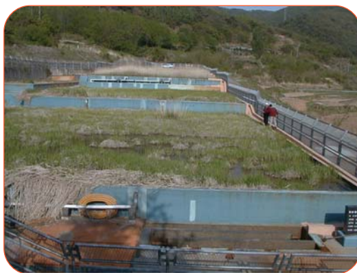
Figure 3: Photograph showing the water treatment ponds with leachate fed by gravity from the acid-generating rock (upper left).
