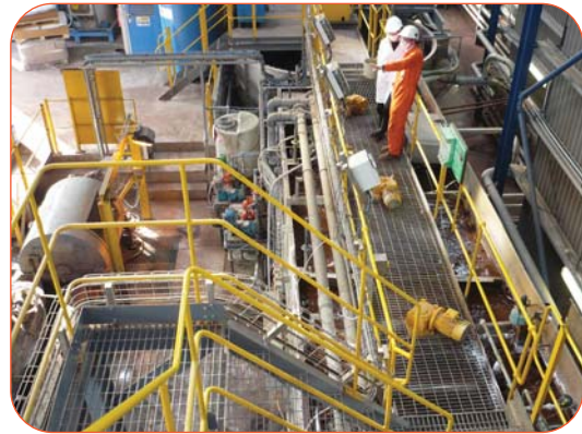
Figure 6: ElectroBind™ was dosed into Tank 1, the first tank at the bottom of this photo; TMT and Amerfloc would be routinely dosed in the next two tanks (seen under plant operators).
