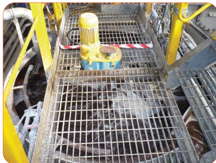
Figure 2: Overhead view of the pre-conditioning tank where raw inlet influent is mixed thoroughly prior to chemical dosing.
