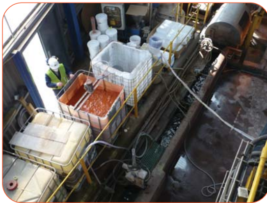
Figure 3: Overhead view of the IBC containing ElectroBind™ and mixer, centre left, and raw inlet work running diagonally from lower left to upper right.
