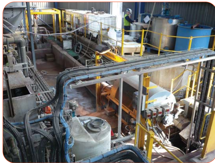
Figure 1: Raw inlet channel running diagonally from top left to centre of photo; ferric chloride is typically dosed in the circular drum, centre, to aid the settling of solids prior to treatment.
