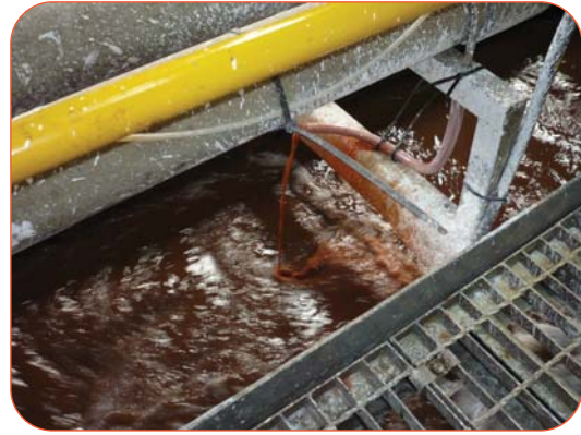
Figure 4: ElectroBind™ being dosed into Tank 1.
