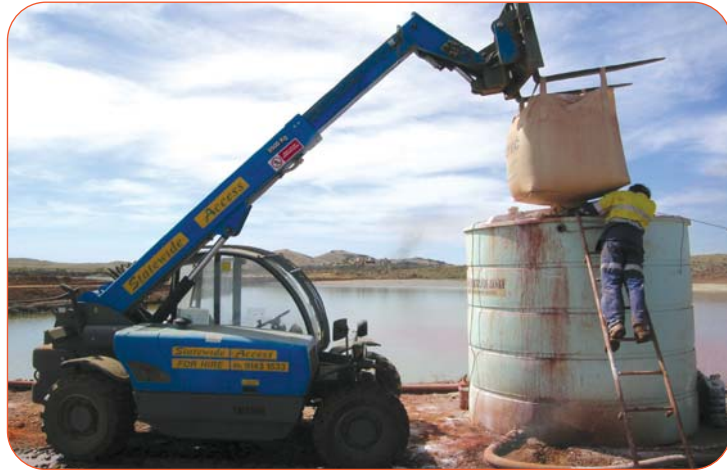
Figure 2: Addition of Acid B™ reagent into a mixing tank to produce a slurry that can be sprayed onto the tailings dam.
