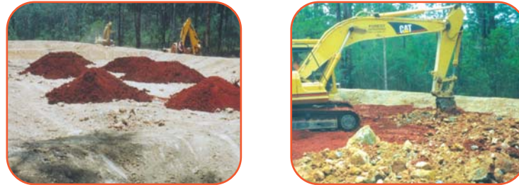
Figure 2. This figure shows the steps taken during the addition of the Terra B™ reagent at Mt Carrington. The site was levelled using the excavator to allow access to the trucks. Terra B™ reagent was transported to the site by truck and deposited in piles. The piles were then spread and incorporated using an excavator. The haul road contained a range of size fractions, from fines to boulders greater than two metres in width (far right).
