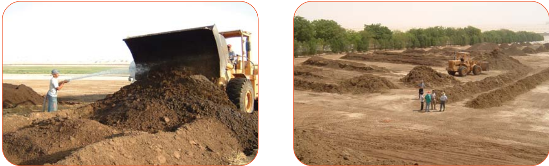
Figure 3 - Mixing of the ViroBlend™ reagent into the waste product (left) Overview of the project area (right)
