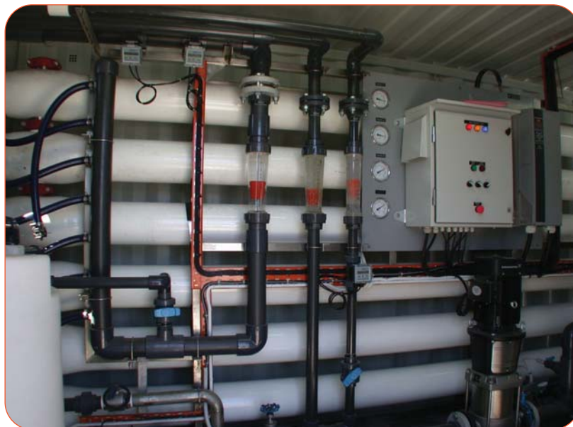
Figure 2 - Reverse osmosis system at the site
