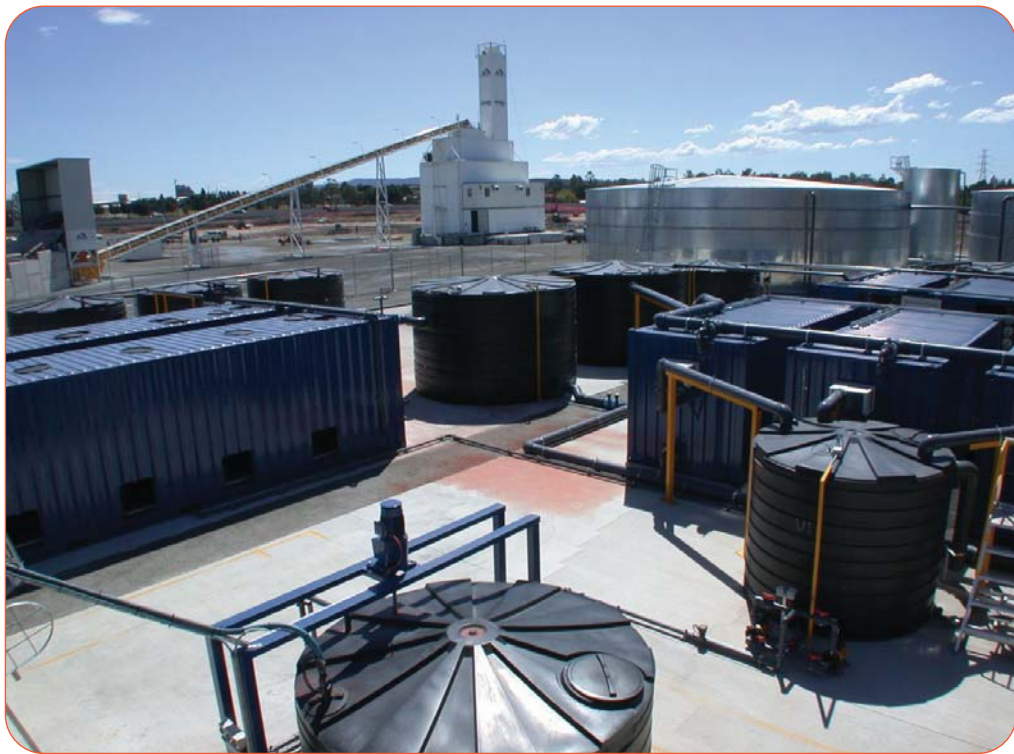
Figure 3 - The groundwater treatment plant at the Origin Alliance site
