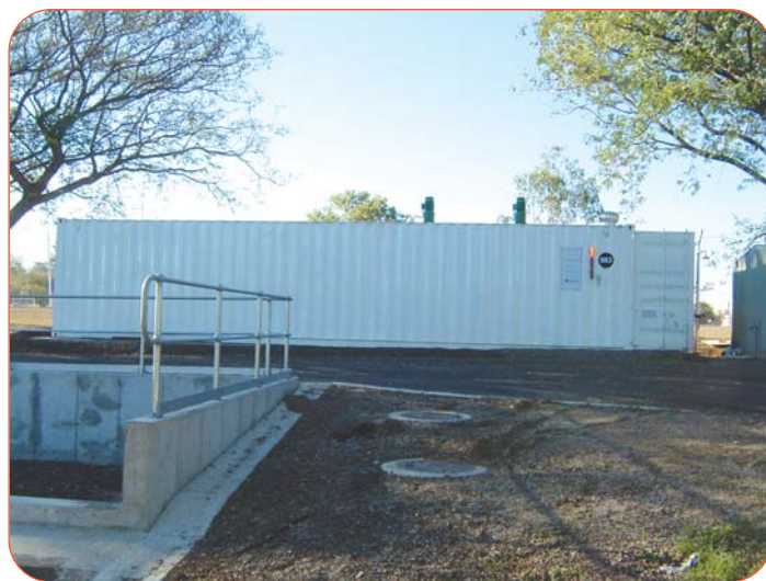
Figure 4: The ViroSewage™ Technology dosing plant at Amberley Sewage Treatment Plant (STP).
