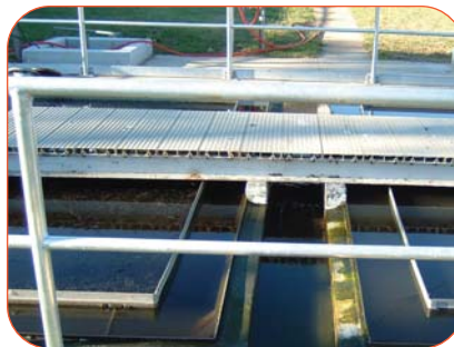
Figure 2: Primary Sedimentation Facility
