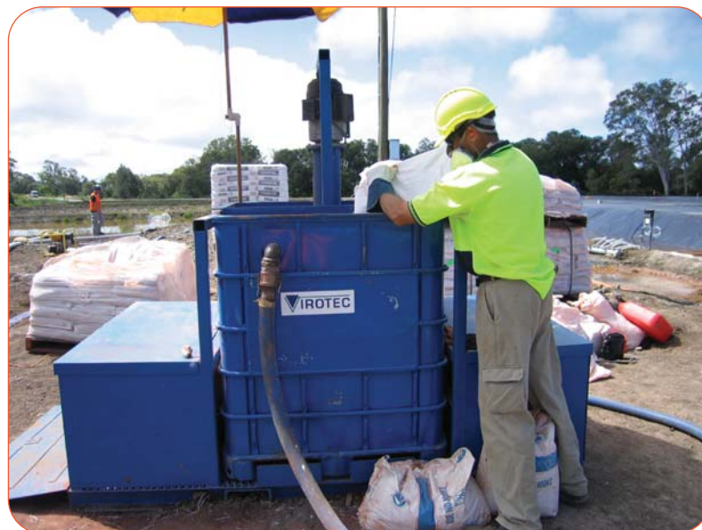
Figure 2: Treatment dosing plant used to mix the ElectroBind™ reagent in with the contaminated water so it can be sprayed back over the surface of the dam.
