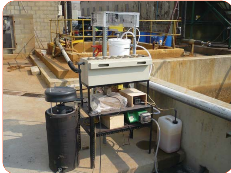
Figure 4: Contaminated site run-off was pumped from the holding lagoon to this ViroFlow™ Technology filter system, which included an iron and acid dosing phase, a solids' settling phase, and a filtration and metal-binding phase.
