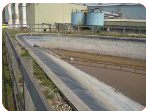
Figure 3: The lined holding lagoon where contaminated site run-off is collected and held prior to treatment by the ViroFlow™ Technology filtration system.
